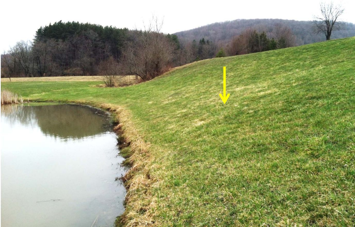
PHOTO 3: CRITICAL TREATMENT AREA (100-FT x 50-FT) LOCATED ON THE NORTH SIDE OF THE STORMWATER POND.
