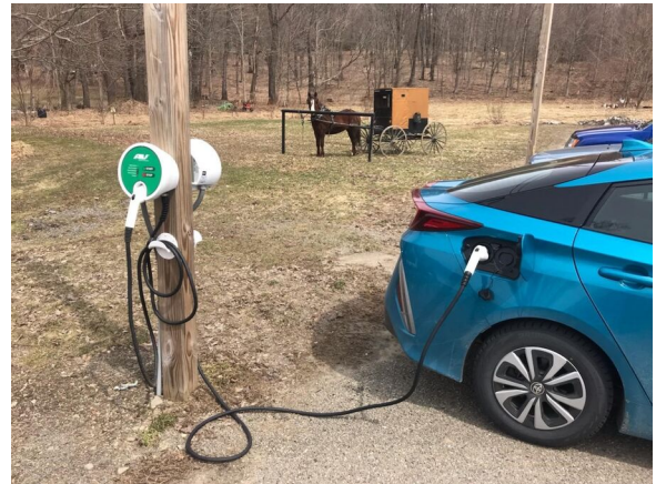
Picture taken at EV charging station in Stockton, NY
