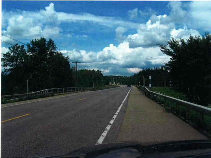
Photograph 37 Looking north on NYS Rt. 60 at a bridge over the Connewango Creek.
