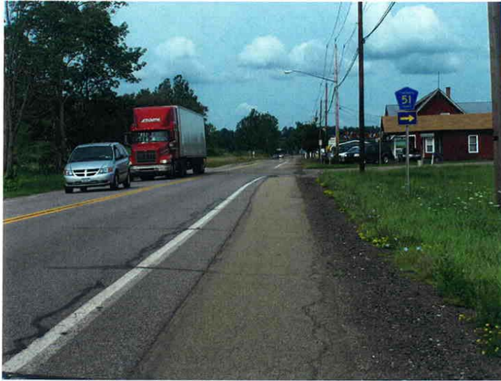
Photograph 3 Looking north on NYS Rt. 60, at the intersection of CR 51. There are two 11.5' wide lanes, one 9' wide tuning lane and 7' wide paved shoulders.
