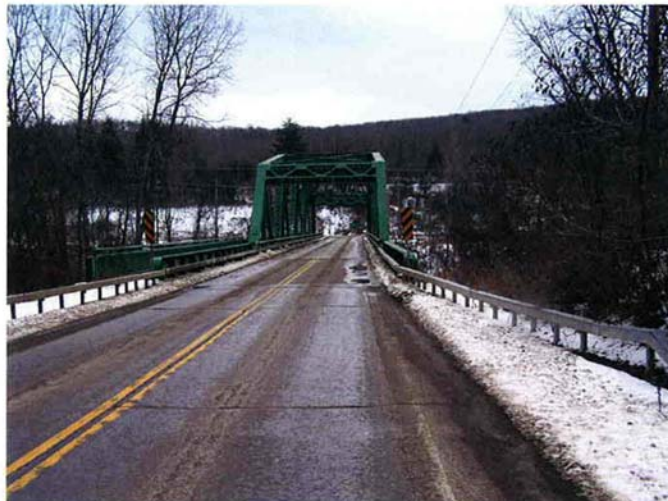
Photograph 4 The Transit Hill Bridge and the intersection of NYS Route 19 and Allegany County Route 16.
