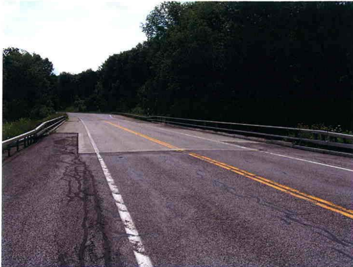
Photograph 35 Looking south on NYS Rout 60 and the bridge over CR 380. The transition to two lane is in the background.
