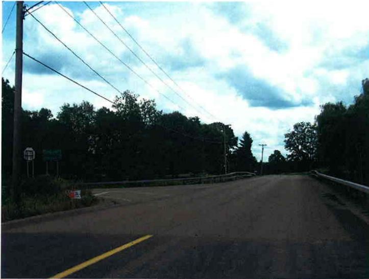
Photograph 10 Looking south on CR 65, at the intersection with Wilson Hollow (4.1 miles south of intersection with NYS Rt. 60). Note the change in pavement in the foreground and the bridge over an unnamed tributary to Cassadaga Creek in the background.
