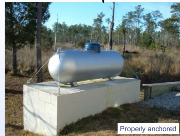
Anchored Propane Tank
